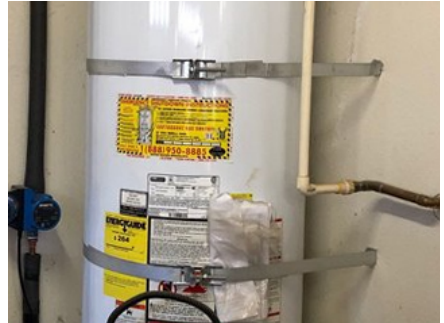
WATER HEATER Two Photos: One of front and one from side with proper strapping
